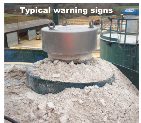
Safety compromised as complete blockage
